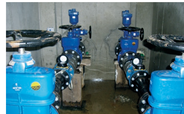
Condition monitoring for slide valves
